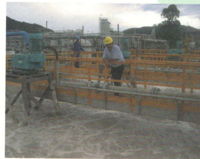
5 HYPERCLASSIC® -Mixing & Aeration Systems in an industrial wwtp in Brazil (Chemical Industry)
